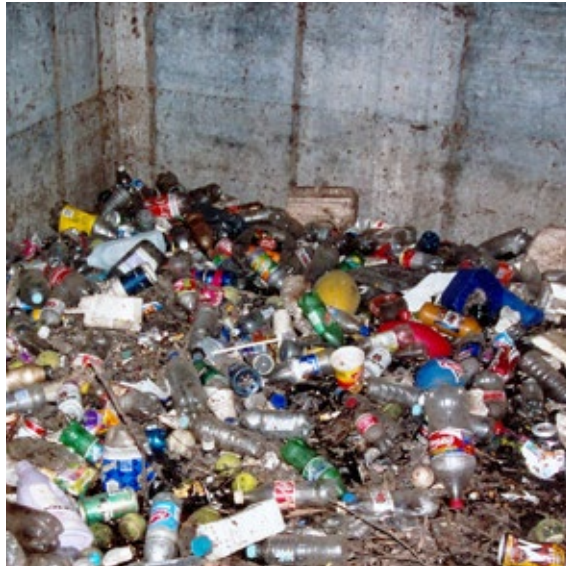
Left: Floating litter captured in the treatment chamber
