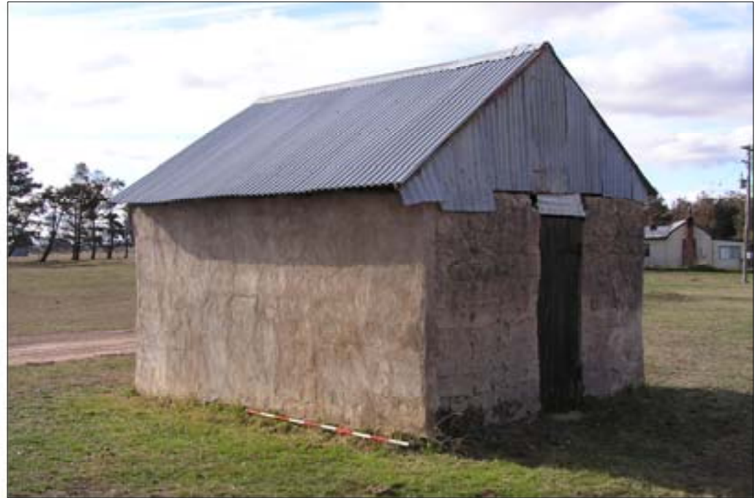
PLATE 2.22 Site MRNH5 External view of southern and eastern elevation of pisé building. Facing NNW. Scale 200mm
