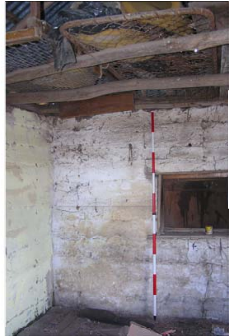
PLATE 2.24 Site MRNH5 Internal view of western wall of pisé building. Scale 200mm
