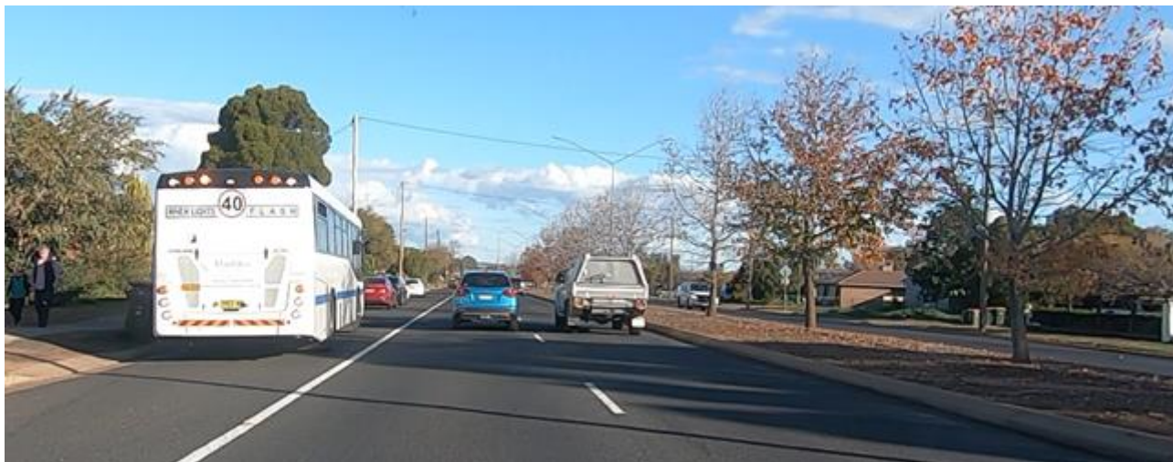
Figure 2.6: Pavement Condition - Northern Section
