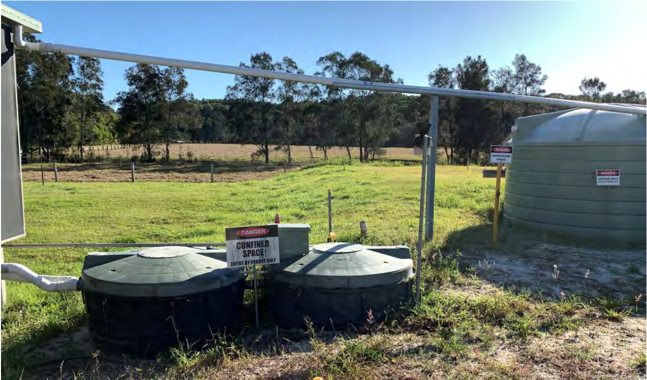
Figure 8 Aerated waste water system, stormwater and signage landscaped areas
