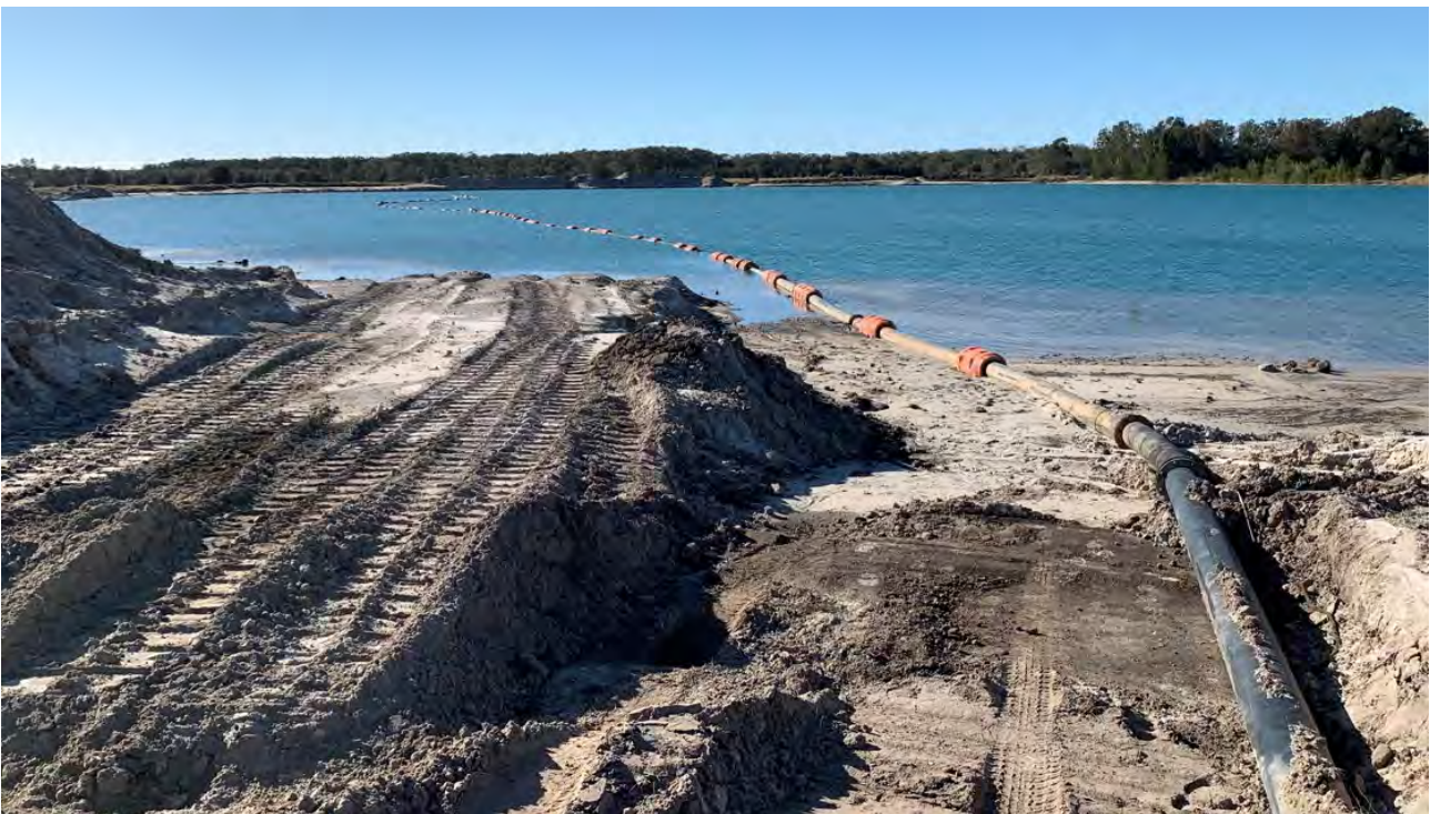
Figure 12 Dredge line from Pond 2
