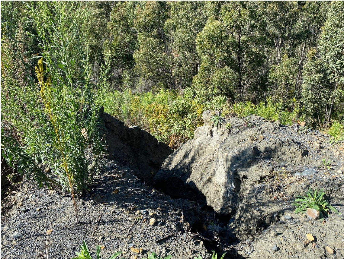
Plate 1 Rill erosion along the outer edge of the Overburden Stockpile area.
