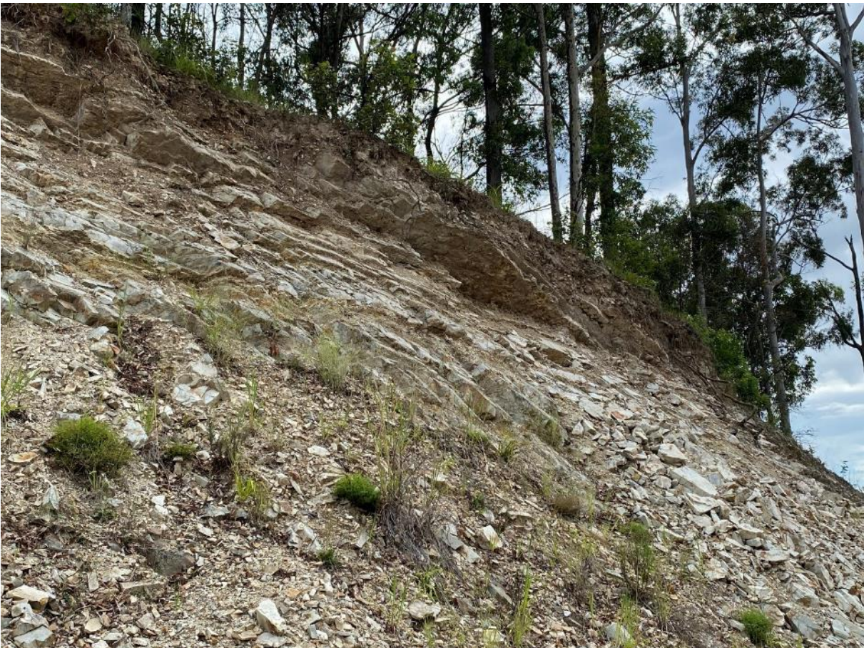
Plate 6 Under-cut from erosion along the high-wall of the western AP area.
