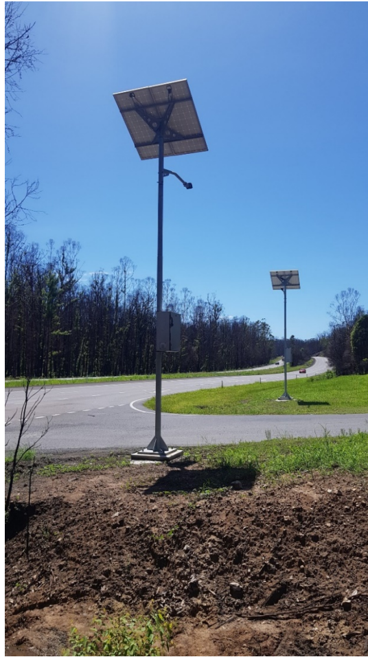
Photo 1: Solar lighting installed at intersection in accordance with Schedule 3 Condition 32.
