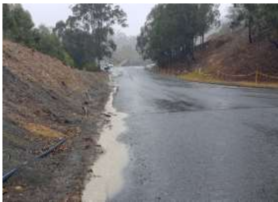
Dirty water observed to be flowing down the Site Access Road, along the western base of the Main Dam, past the LDP
