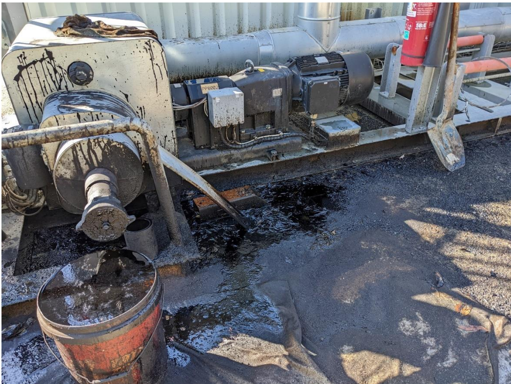
Minor hydrocarbon leakage, primarily on to geofabric, within the Downer plant area
