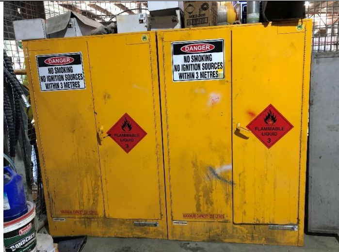
Chemical Storage cabinets within locked, bunded shed
