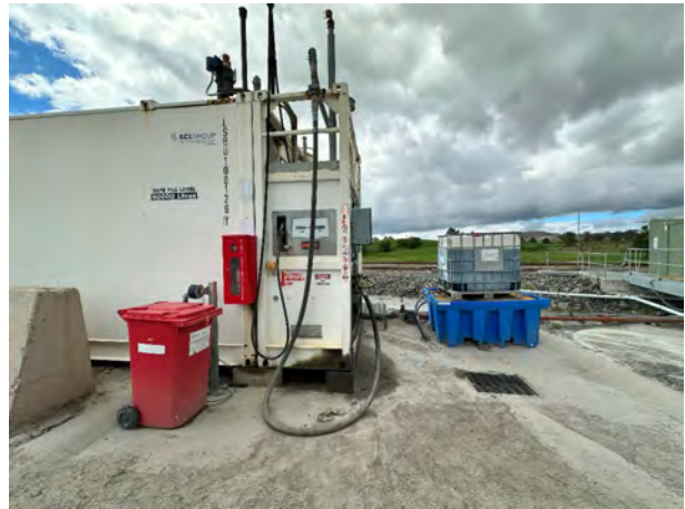
Photograph E.44 Refuelling facility
