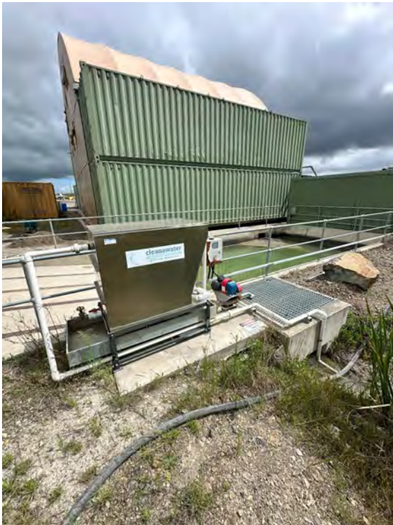
Photograph E.27 Sump oily water separator
