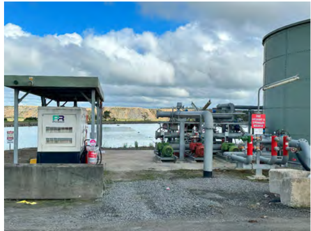
Photograph E.4 Pump station
