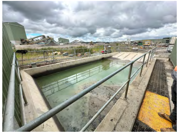
Photograph E.26 Sump
