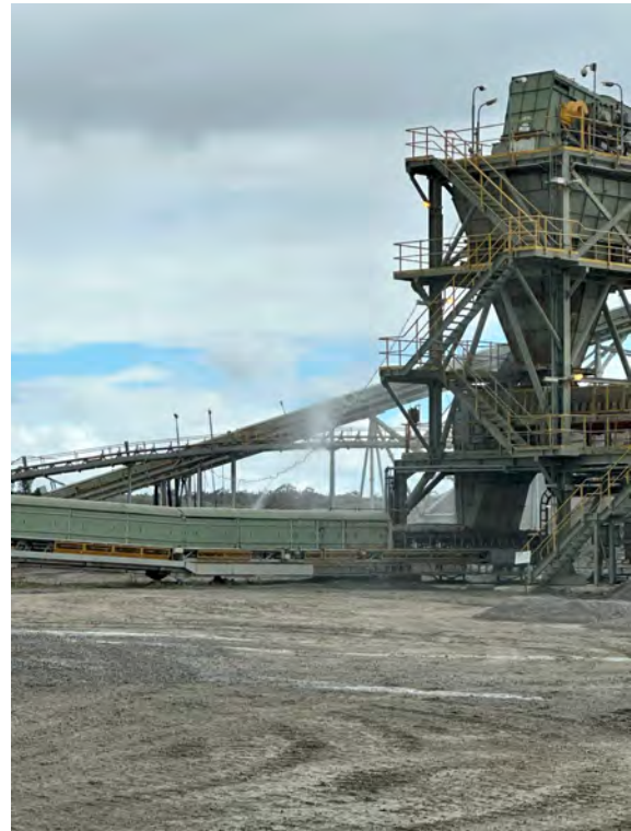
Photograph E.38 Active water sprays on processing facility
