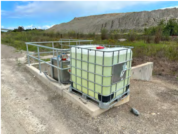
Photograph E.43 Dust suppressant and associated pump
