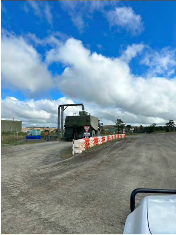
Photograph E.1 Water fill point
