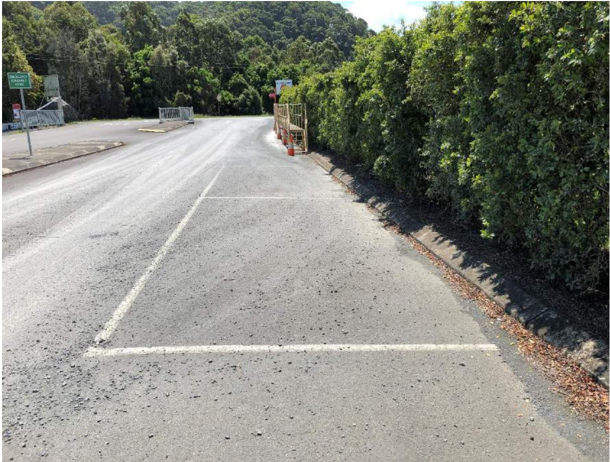
Photograph 13: Main entrance driveway, kerb shown to left of photograph which contains and directs runoff towards weighbridge and truck wash area
