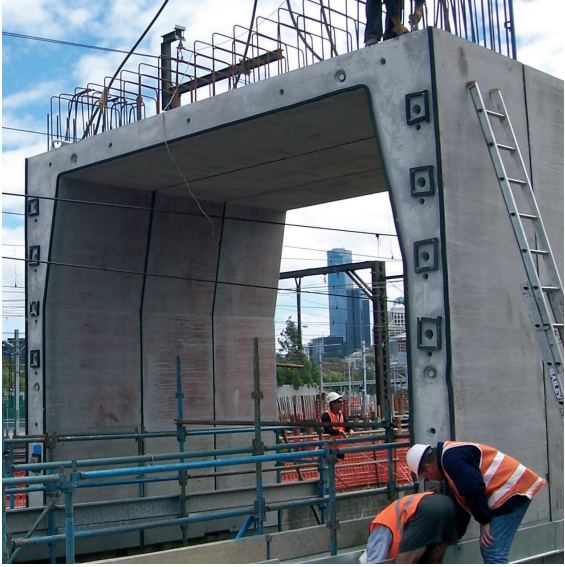
Box culverts with post-tensioning ducts
