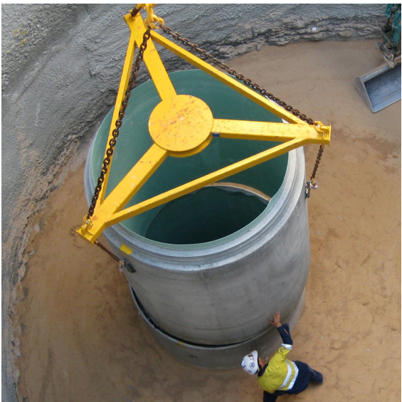
HDPE lined access chamber
