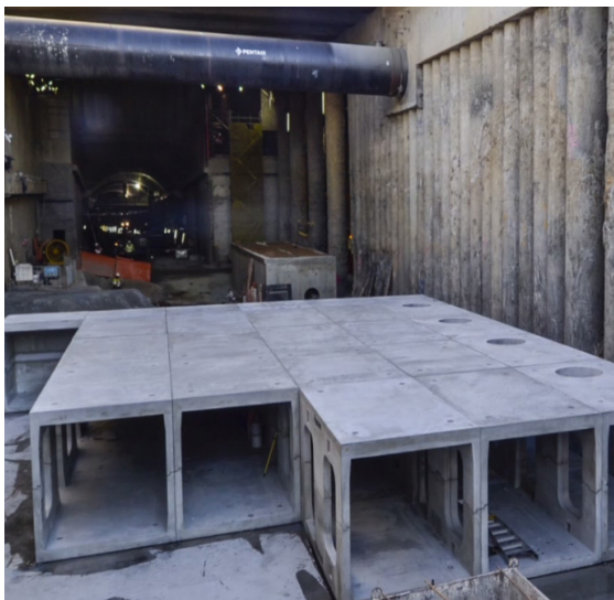
Top: StormTrap® detention system – Legacy Way, Brisbane
