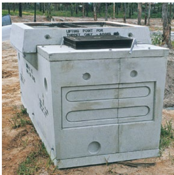
Top: Cable jointing access chamber
