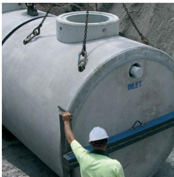
Top: Storage tank
