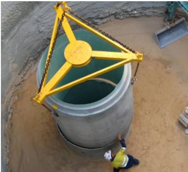
HDPE lined access chamber
