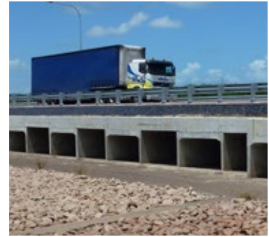
Box culverts - large 51
