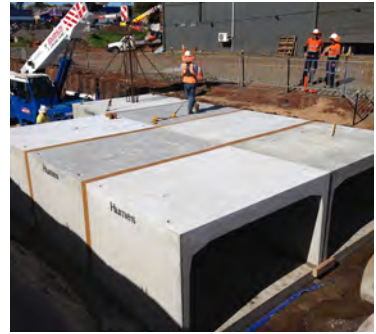
Box culverts - small 14
