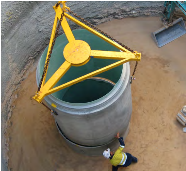
HDPE lined access chamber
