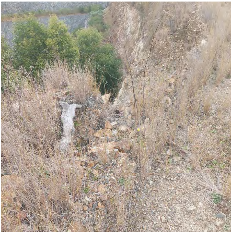
Plate 6 Under-cut from erosion along the high-wall of the western AP area.
