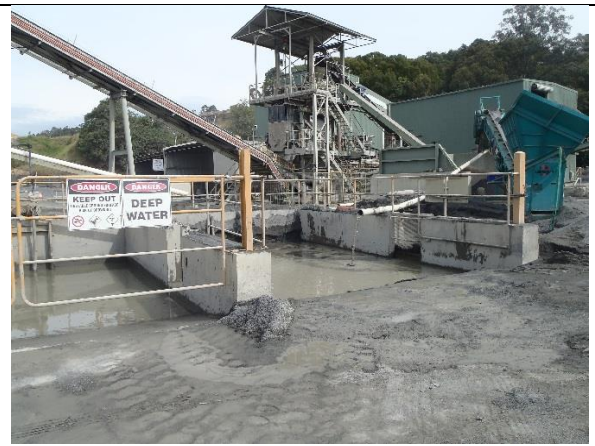
Tertiary crusher and screen, and wedge pits receiving operational runoff from the processing plant. Water is reused in the wet processing plant operation, with excess water pumped to the Main Dam.
