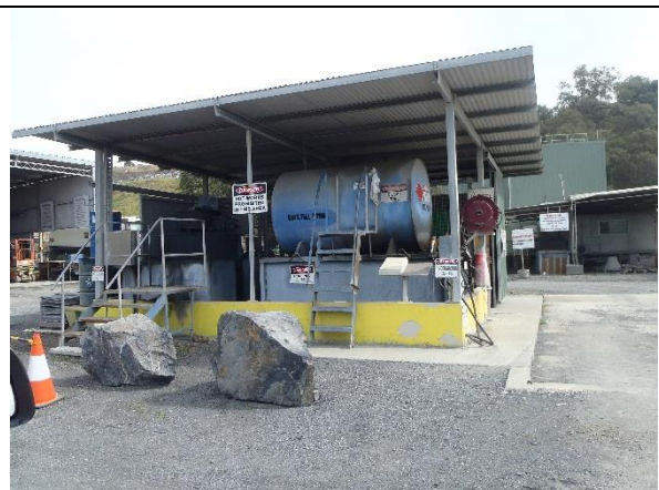
Liquid storage facilities, located within bunding.
