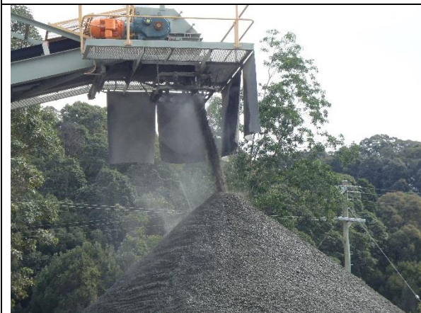
Secondary crusher and screen, with water sprays occurring to minimise dust issues.
