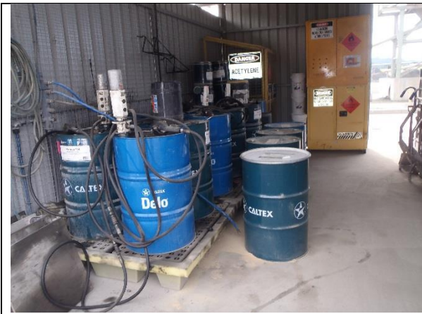
Oil storage, located within bunding.
