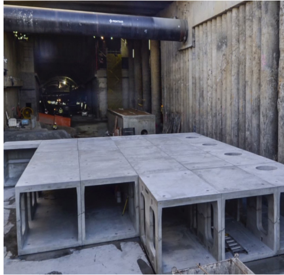
Top: StormTrap® detention system – Legacy Way, Brisbane
