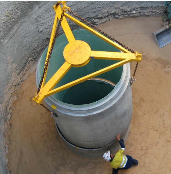
HDPE lined access chamber
