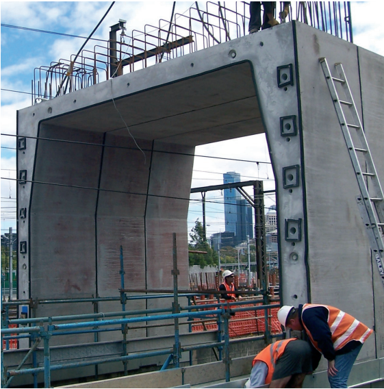
Box culverts with post-tensioning ducts
