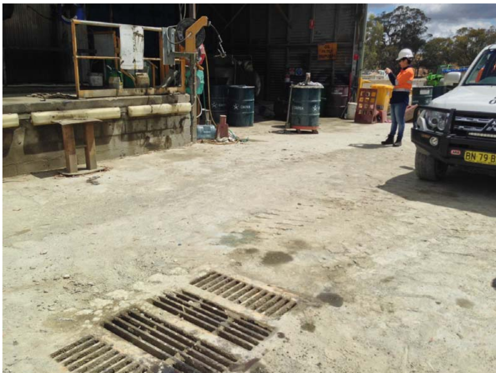
Photograph 5.4 Vehicle maintenance area – drain to an oil-water separator (27/11/14)
