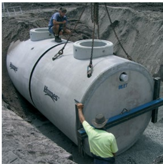
Left: Precast storage tank
