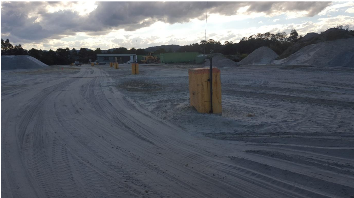
Photograph 4: Sprinkler dust suppression system positioned on bollards.
