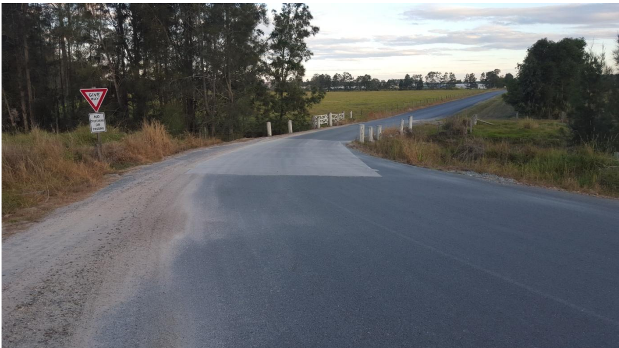
Photograph 6: Sealed haul road with evidence of recent repair work.
