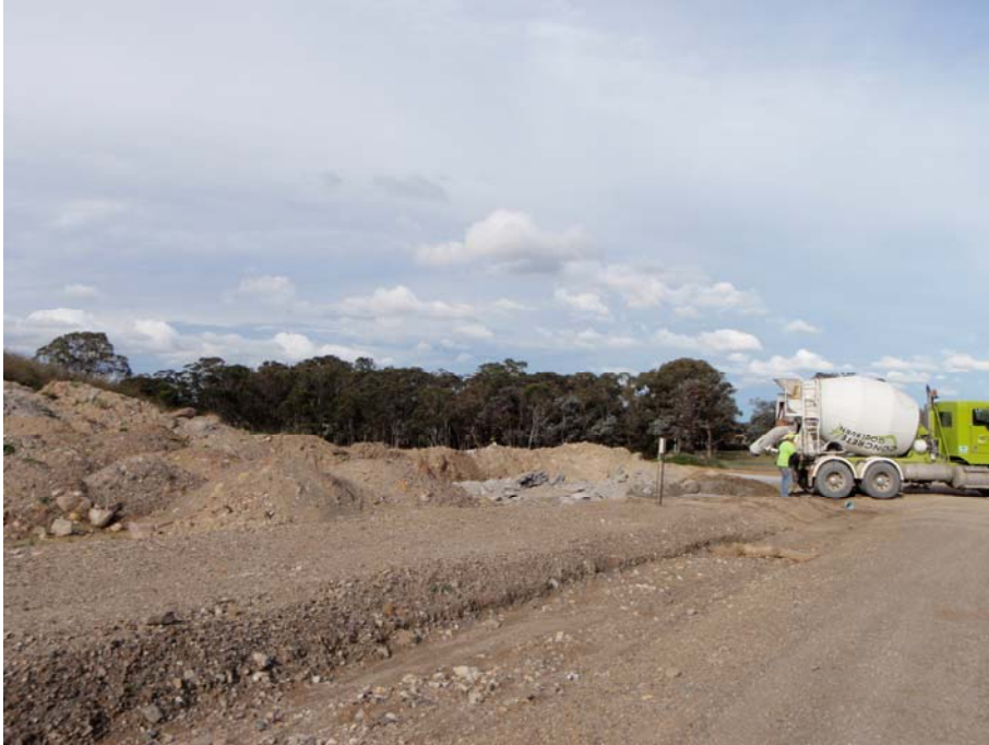
Photograph 5.2 Mixed soil, overburden and waste concrete stockpile south of the Hume Highway intersection construction site (23/4/12)
