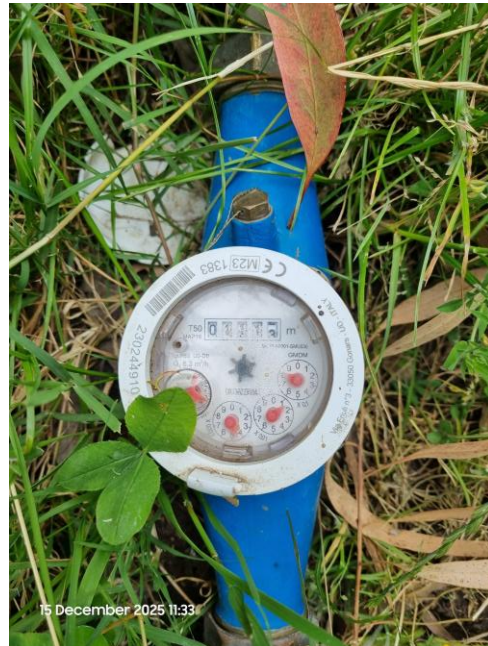
SP02. Flow meter reading of 1,113 m³
