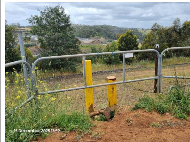
Bore MB01 located at top of steep slope. Slight movement in monument cover noted
