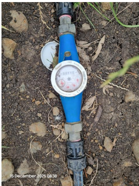
SP03. Flow meter reading of 210.5 m³
