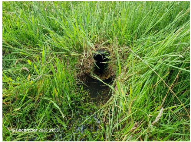
SP08. Culvert and PVC pipe
