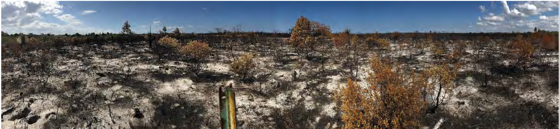
Plate 4: Block I - looking south showing the extent and intensity of the fire on this block (PP12)
