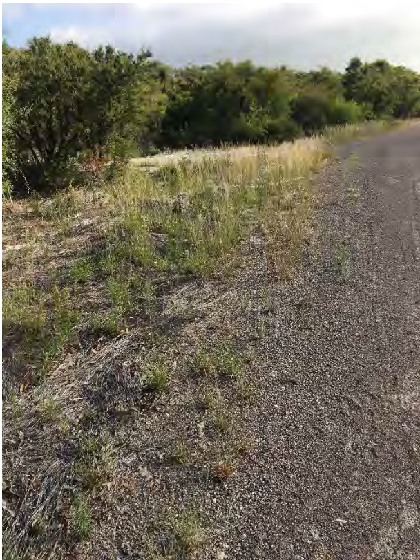
Figure 2 Roadway Weed Growth
