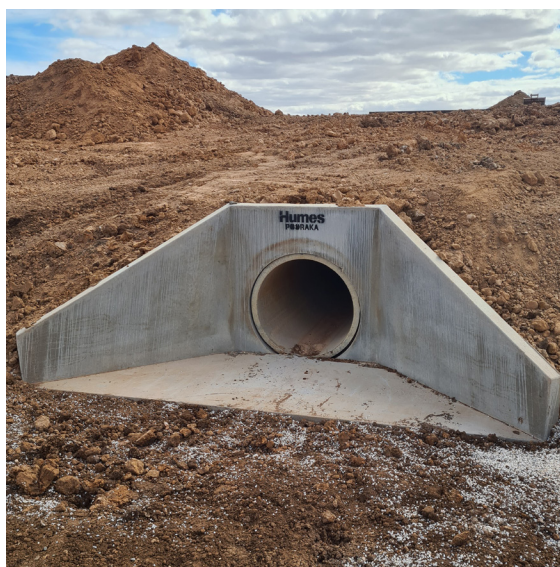
Top: Single steel reinforced concrete pipe headwall
