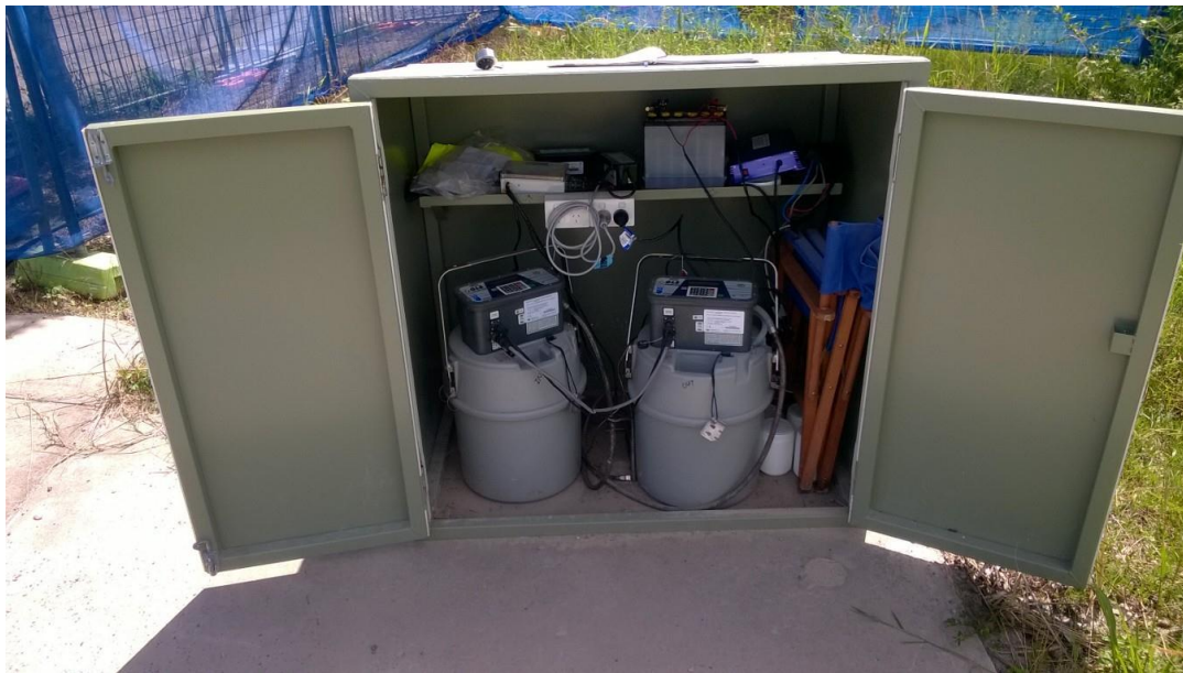
Figure 3 – Steel Monitoring Equipment Housing Installed on Lid of HG27
